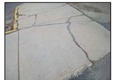
Arlington Street Cracked Sidewalk (1G)
