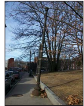
Damaged streetlight (8F)
